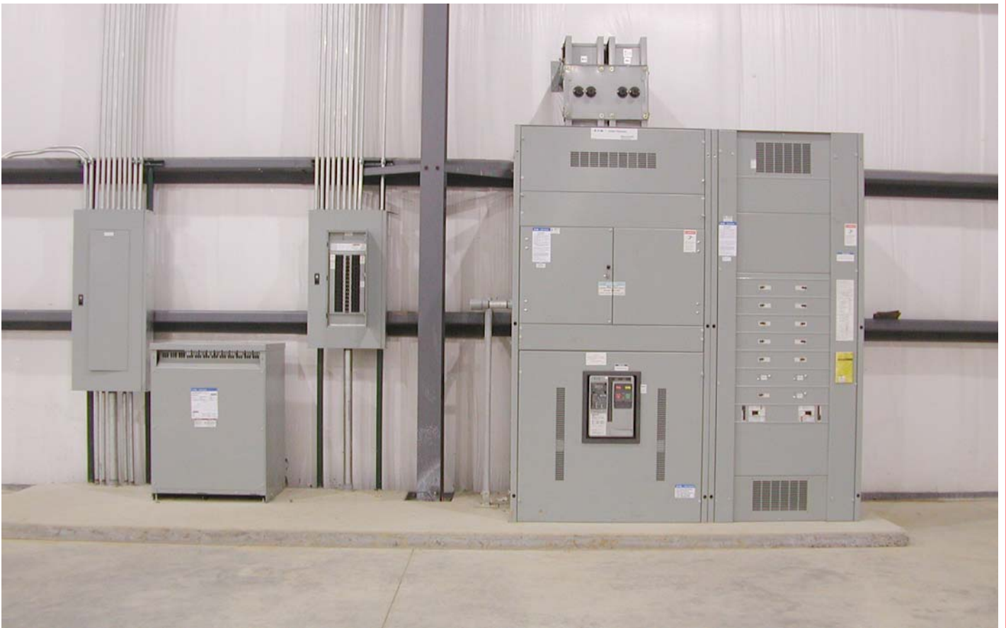
ELECTRICAL SERVICE PANELS
